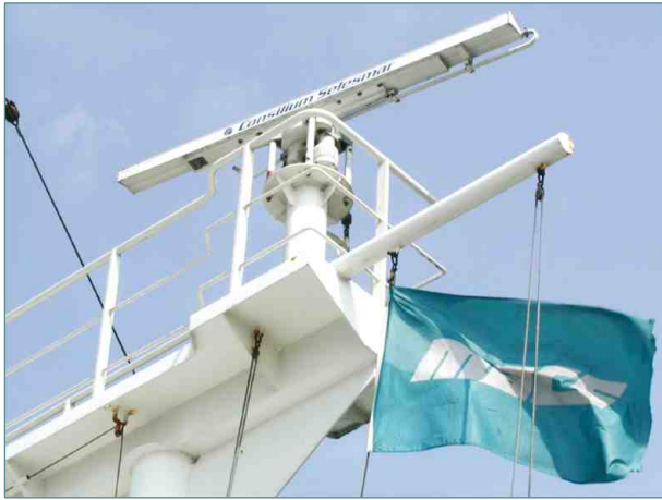
▲ Figure 6 Typical installation of an antenna of a X-band marine radar system.
