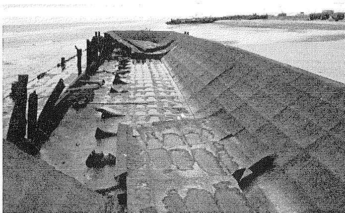
Fig. 4. Pechora Sea coast near the constructed pipeline "Varandei sea". During the winter of 1999-2000 the offshore side of the barge-pontoon was destroyed by fast ice moving rapidly onshore
