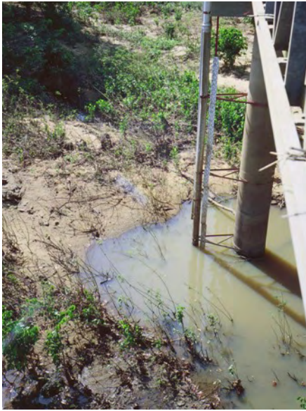
Fig. 8.8 Stagnant water around the turbidity probe at the Terou-Igbomakoro outlet (11/2005).
