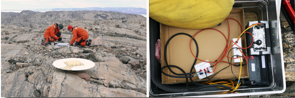
Fig. 8.2: Set-up details of a GNSS station. Left: The GNSS antenna (directly fixed to the rock by a special bolt). Right: View into the Zarges aluminium box with charging controller (centre), GNSS receiver (black case) and a sealed battery (upper right).
