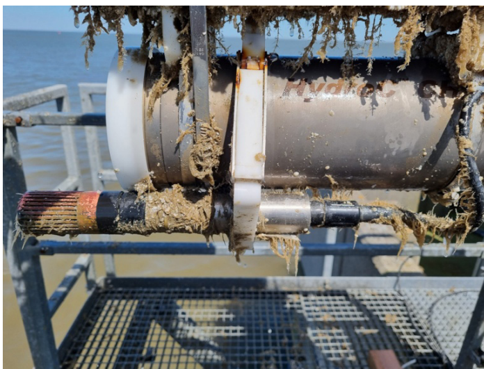
Fig. 5.5: Methane sensor 4 weeks after deployment in Cuxhaven; photo: I. Bussmann
