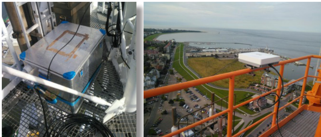
Fig. 9.2: ZargesBox containing all modules for the land station (left) and the antenna mounted approx. at a height of 90m a.s.l. in the direction of the German Bight (right); photo: P. Sprich, WSA
