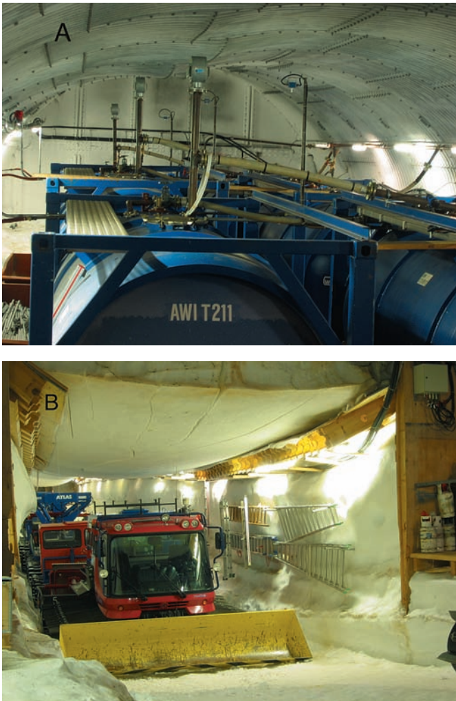
Fig. 19: Deformation of Neumayer Station II in the 13th year of its existence. A = View into the 92 m long cross tube, where the diesel tanks are mounted. The deformation of the tube, caused by the permanently increasing load of accumulated snow, can clearly be seen. B = View into the tunnel connecting the tube system with the garage. To keep a sufficient tunnel height, the compressed snow has to be cut out every third year.
