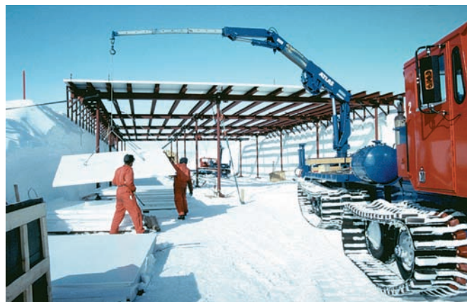
Fig. 18: The innovative garage trench at NM-II under construction. The roof can easily be lifted up and the garage floor backfilled with snow in accordance with yearly snow accumulation while the garage remains accessible through a tunnel with the station tubes.
