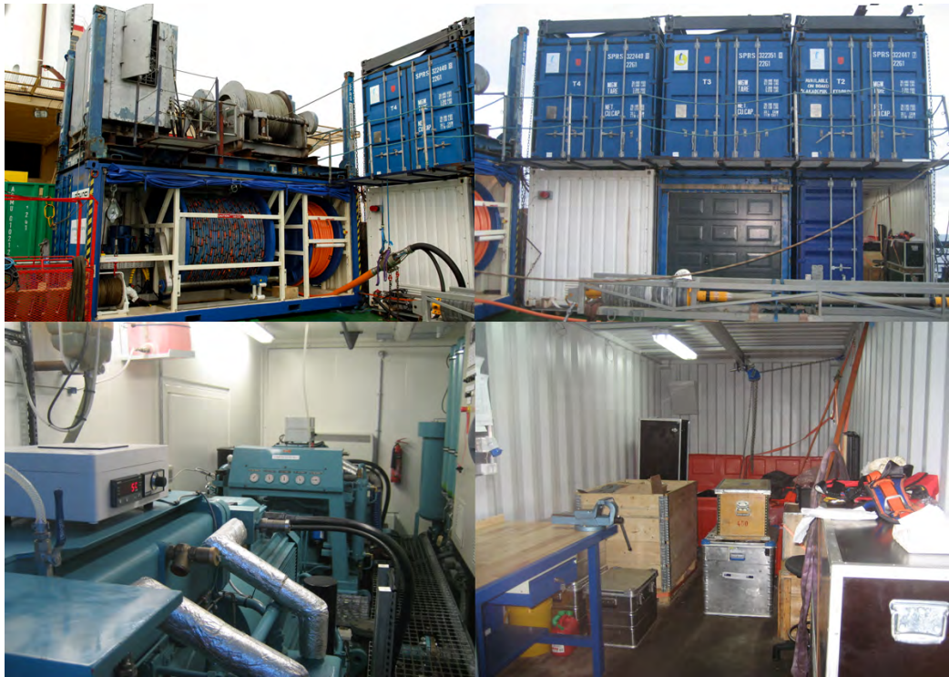
Photos 19-22. On top the winch container and workshop container with storage containers above. Below interior of compressor and workshop container.
