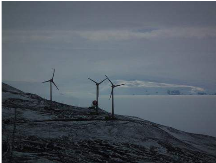
Figure 3.9. Wind turbines on Ross Island, Antarctica, providing power to the US McMurdo Station and the New Zealand Scott Base (© D. Liggett, 2014)
