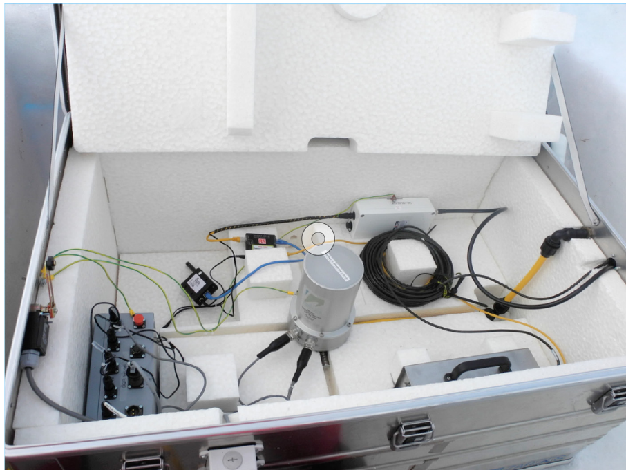
Fig. 4.4.3 The insulated field-box contains the microbarometer (in the middle), data acquisition system as well as the power supply and a communication unit
